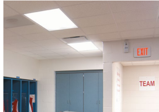
Exit and Emergency
